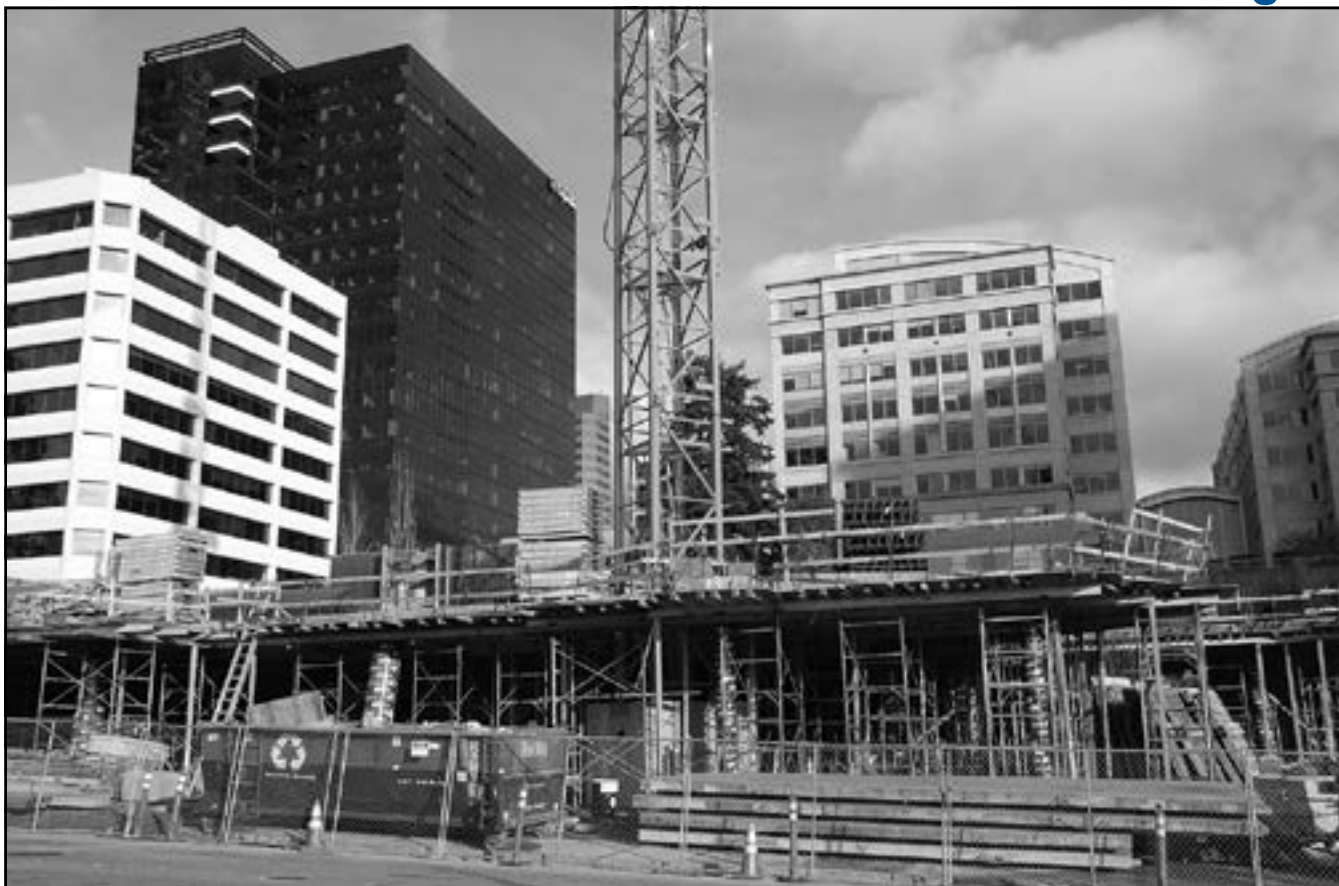
The only tower crane in downtown Bellevue is at the construction site for Soma Towers, a 266-unit apartment complex being built at Northeast Second Street and 106th Avenue Northeast. More cranes may be on the way.
