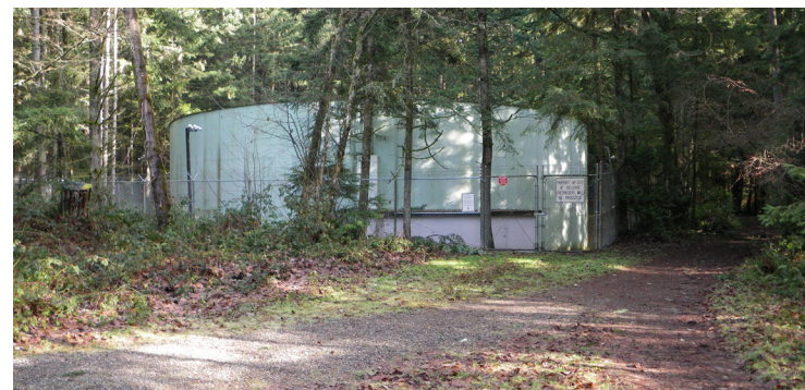
Pikes Peak Reservoir and Pump Station
