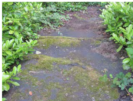
Change in level in an asphalt sidewalk at SE 27th Street & 124th Avenue SE.
