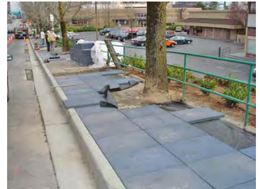
Rubber sidewalk panels at NE 10th Street west of 102nd Avenue NE allow tree roots to grow under the sidewalk without creating a change in level barrier for people with disabilities.
