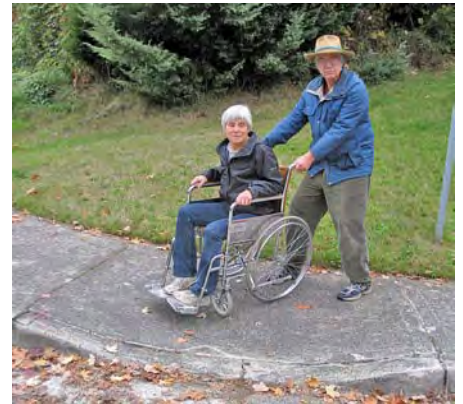
No ramp landing panel.
