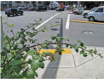
Encroaching vegetation on ramp.
