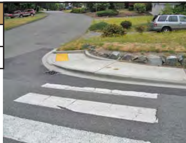
Ramp not aligned with crosswalk at Main Street & 164th Avenue NE.
