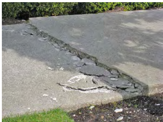
Two inch change in level in a concrete sidewalk at 58th Place & SE 58th Street.
