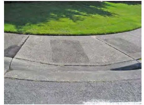
Missing detectable warning surface.
