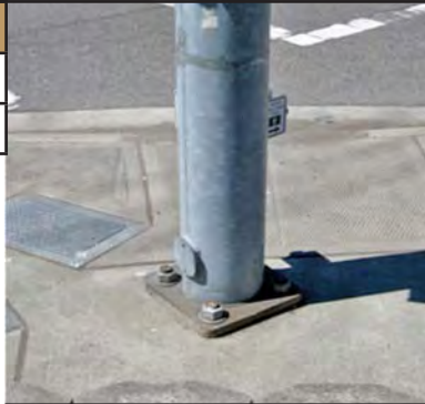
Obstruction in ramp landing panel at SE 36th Street & Factoria Boulevard SE.
