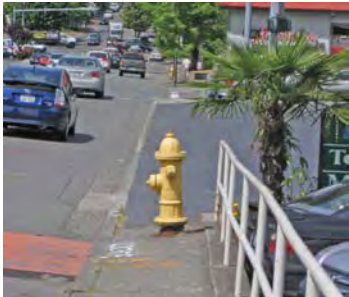
Hydrant on 3 foot sidewalk at Main Street & 107th Avenue NE renders sidewalk unusable to people with disabilities.
